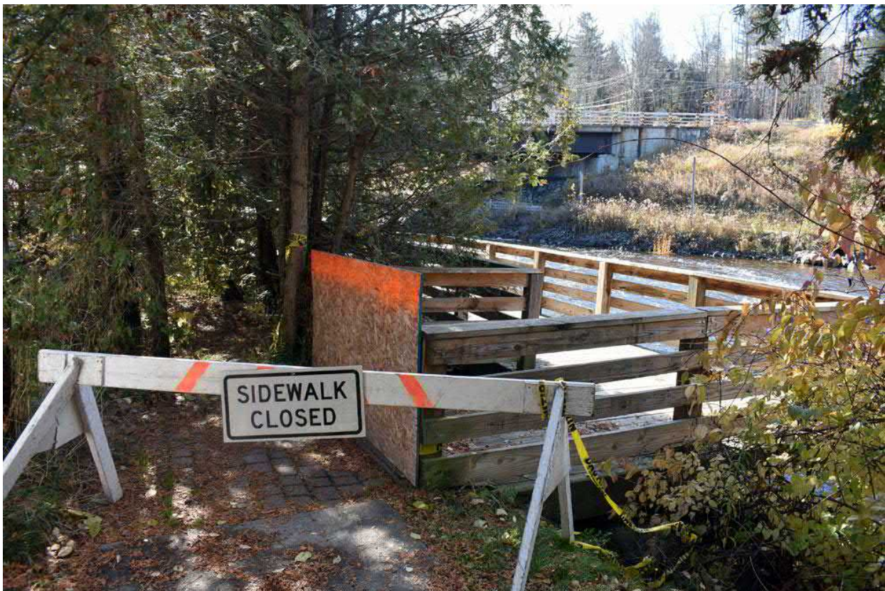
Part of the Saranac Lake River Walk was closed in October for repairs. Village Mayor Clyde Rabideau said it will stay that way through the winter. (Enterprise photo — Griffin Kelly)
